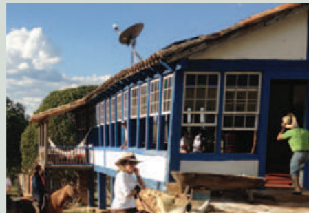
BOA VISTA – The structure of this early 19th century house was strengthened and it received a new porch and some functional updates. Everything was with architectural preservation in mind.
